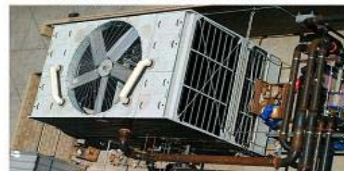
Cooling Tower for AD & Fuel Cells
